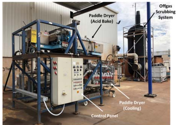
Figure 2: Large scale Phase 4 Acid Bake Pilot
