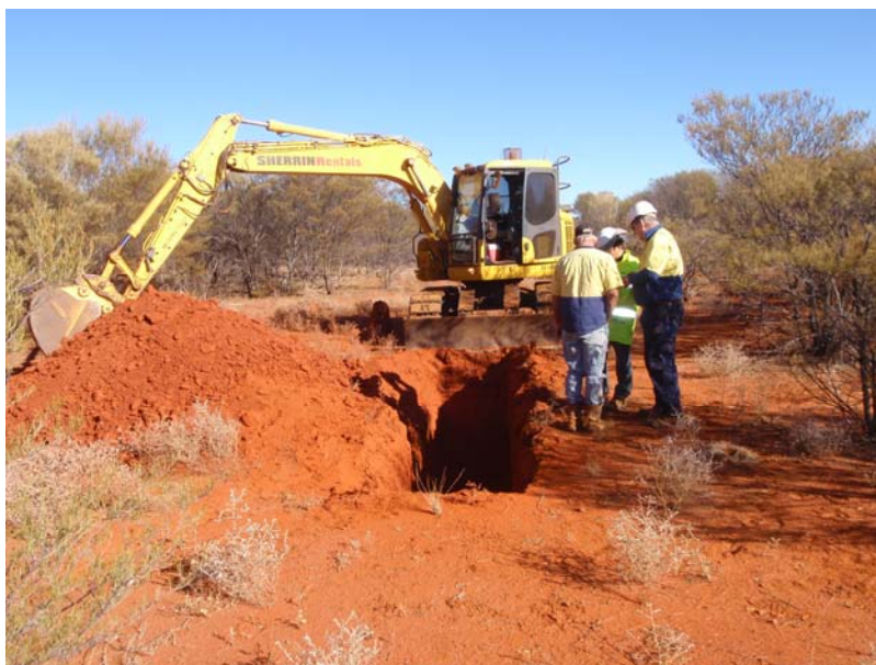
Geotechnical test pit excavation at the site of the Nolans process plant
