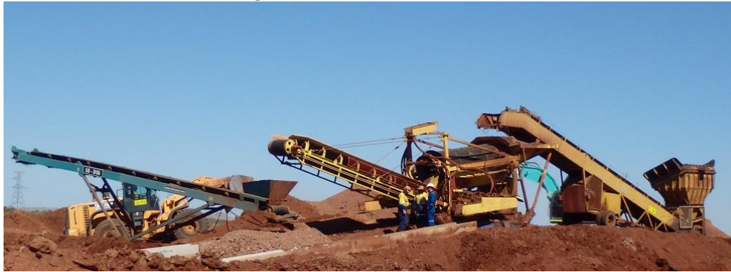
Figure 1: Nickol River Gold Processing Plant:
