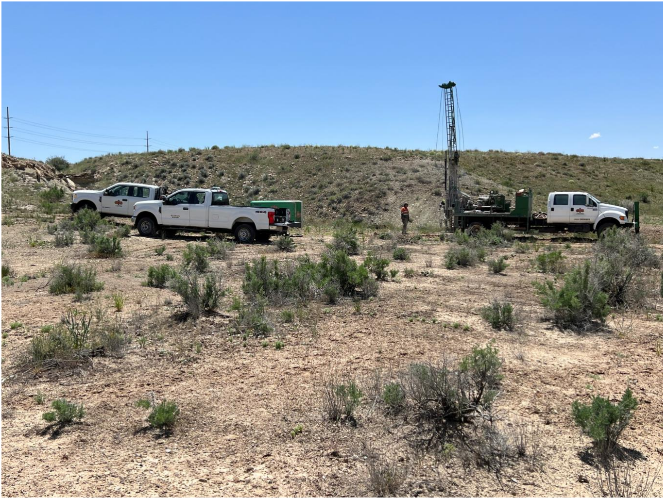
Figure 1: Photo showing the drilling rig on site carrying out geotechnical engineering work. Powerline infrastructure within the property is also shown.
