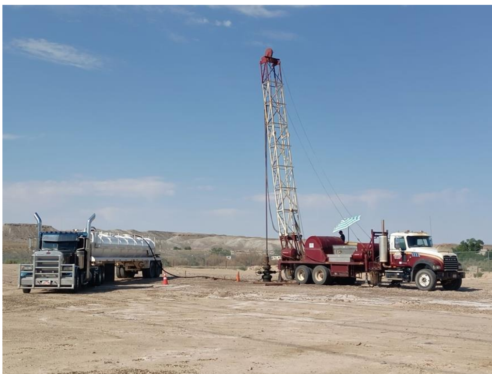
Figure 1: The “swabbing” truck collecting brine samples to be taken to the Koch DLE Extraction Pilot Unit
