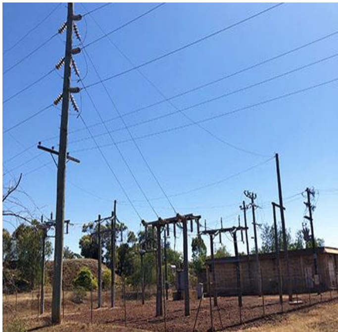
66 kVA electricity sub station already on site at Sconi
