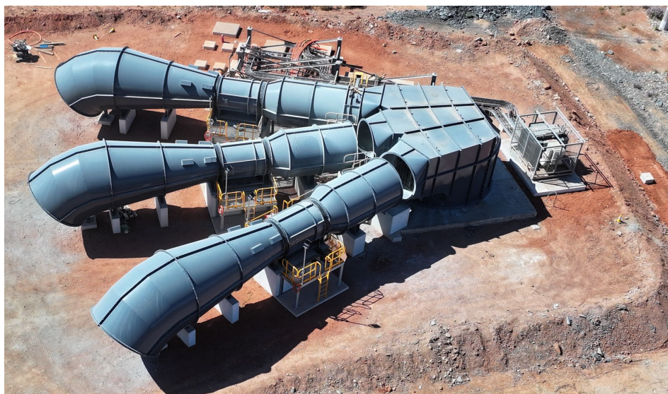
Figure 2: Underground primary ventilation upgrade installed and due to be commissioned commencing 18 September 2024.
