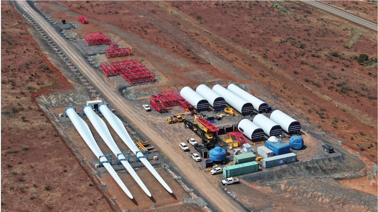
Figures 7 & 8: Crane on site and being put together for construction of the 4 x 6MW wind turbines, to be completed by H2 FY25. All components on site and ready for installation.
