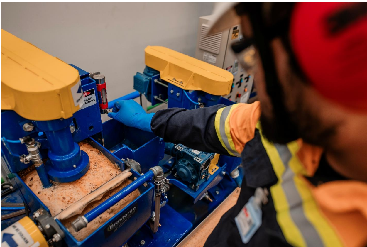
Figure 10: Flotation cell air flow adjustment during commissioning.
