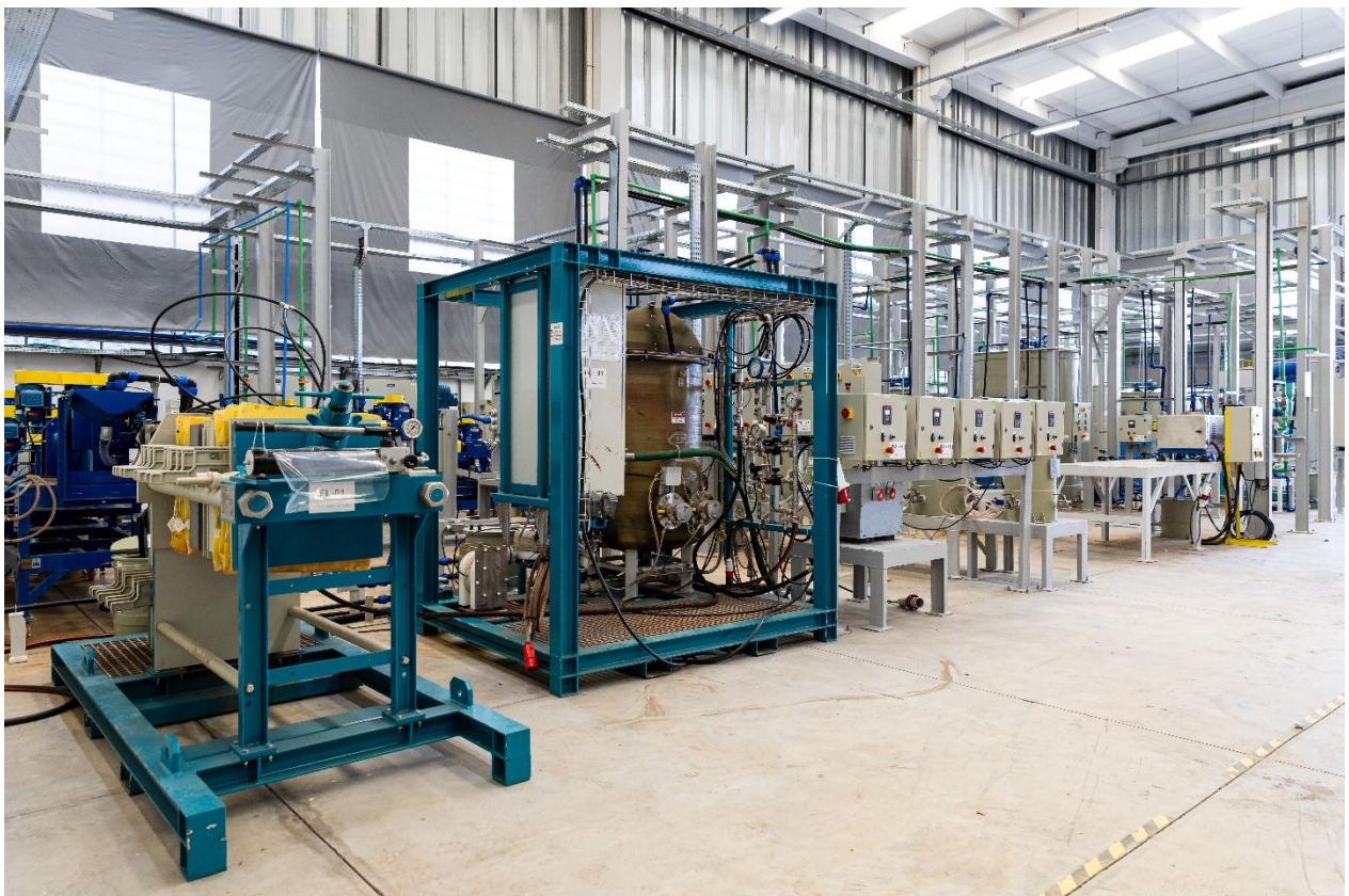
Figure 13: Filter press in the foreground, providing solid-liquid separation.
