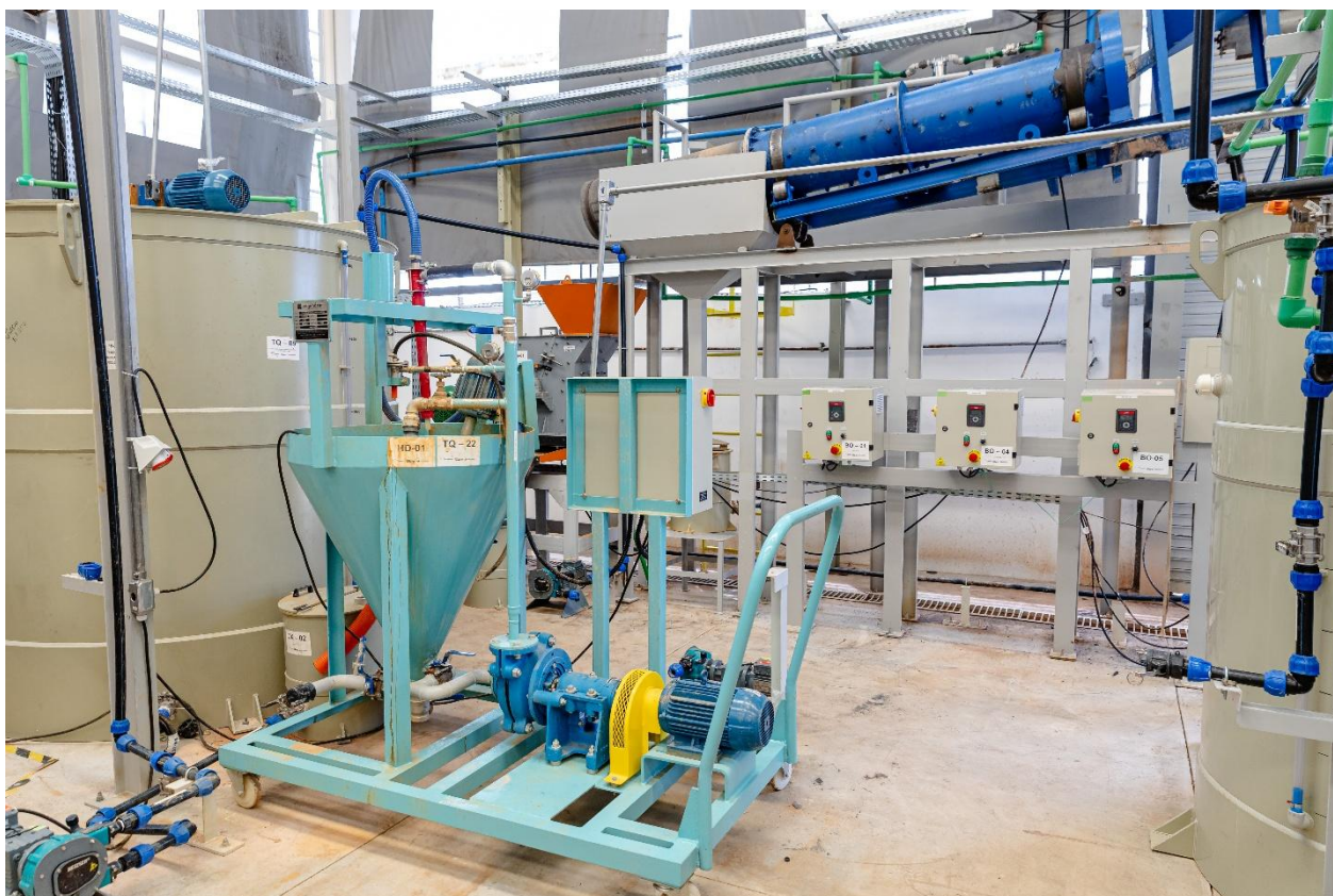
Figure 6: Hydrocyclone classification equipment and associated slurry tank and pump.
