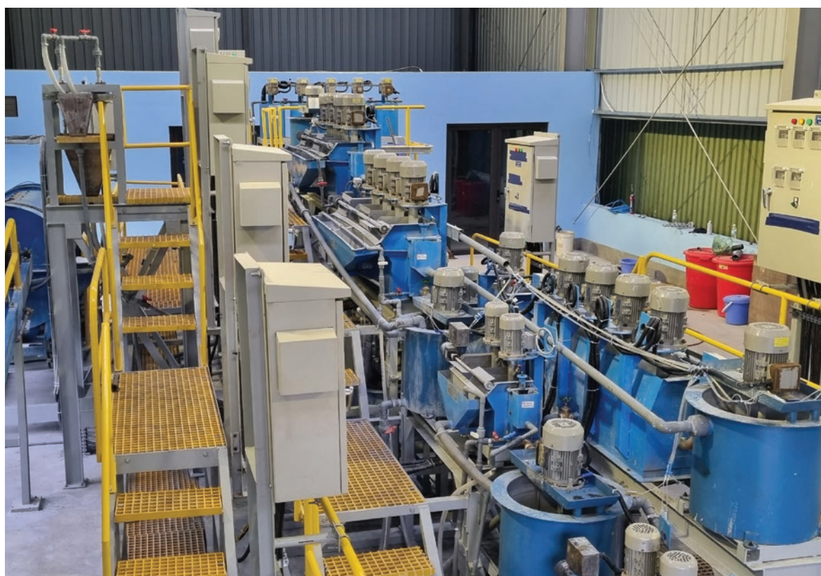
Figure 9 - TKN Pilot Plant located at the mine site
