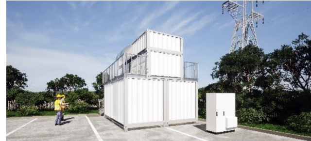
Trial project for Energex in Queensland using a Sumitomo Electric Industries vanadium battery 250 kW / 750kWh
