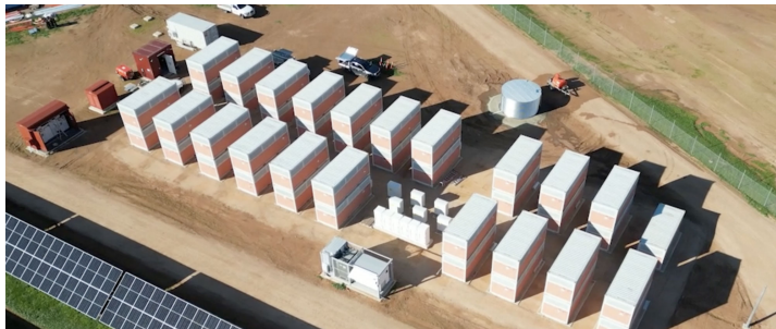
Bungama, port Pirie, South Australia 2MW/ 8MWh Vanadium Flow battery
