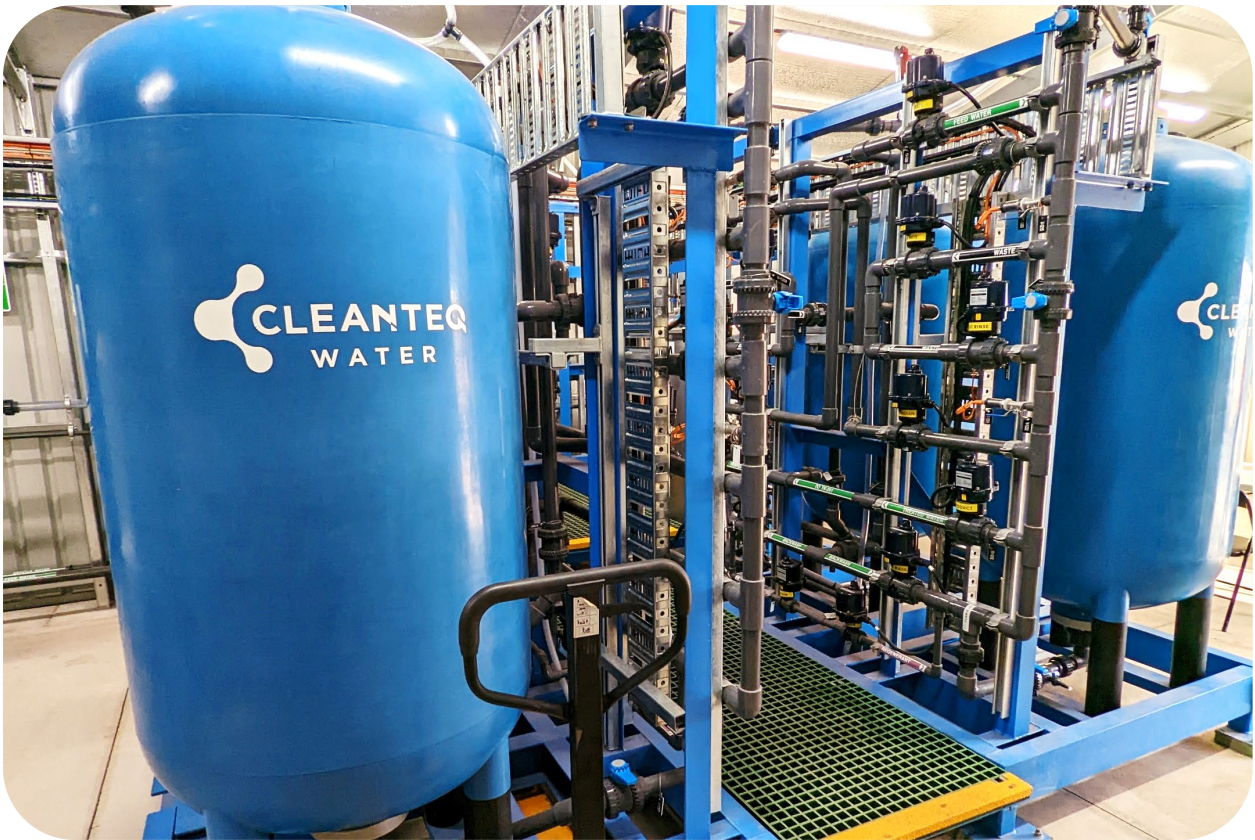
Photo of the two skid mounted batch ion exchange systems at Laramba
