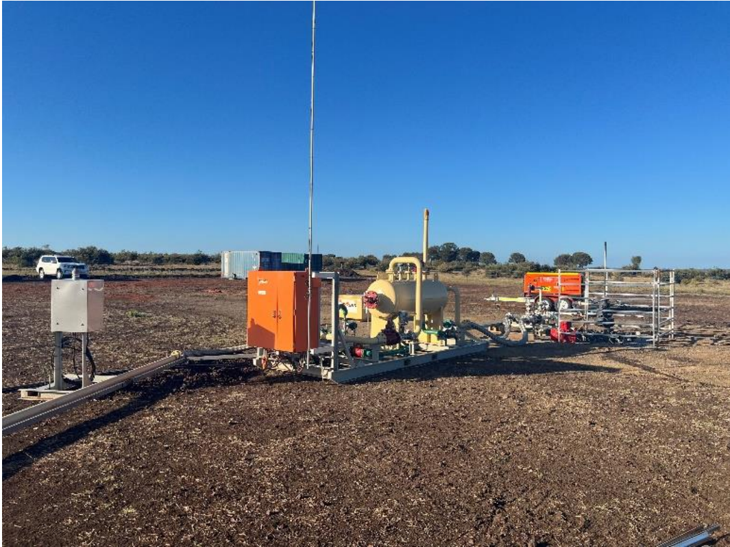
Figure 1: Mahalo East 1 vertical well connected into production separator and metering skid
