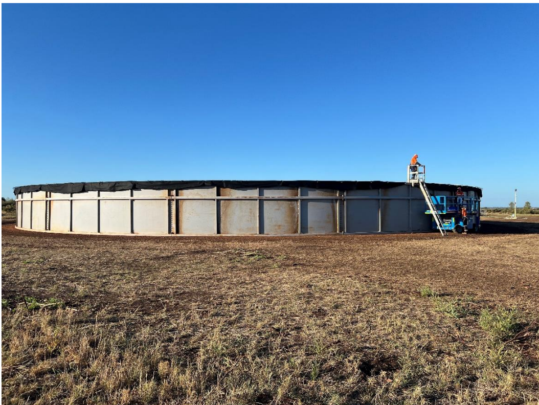
Figure 2: Mahalo East water storage tank installation with flare stack in background on right
