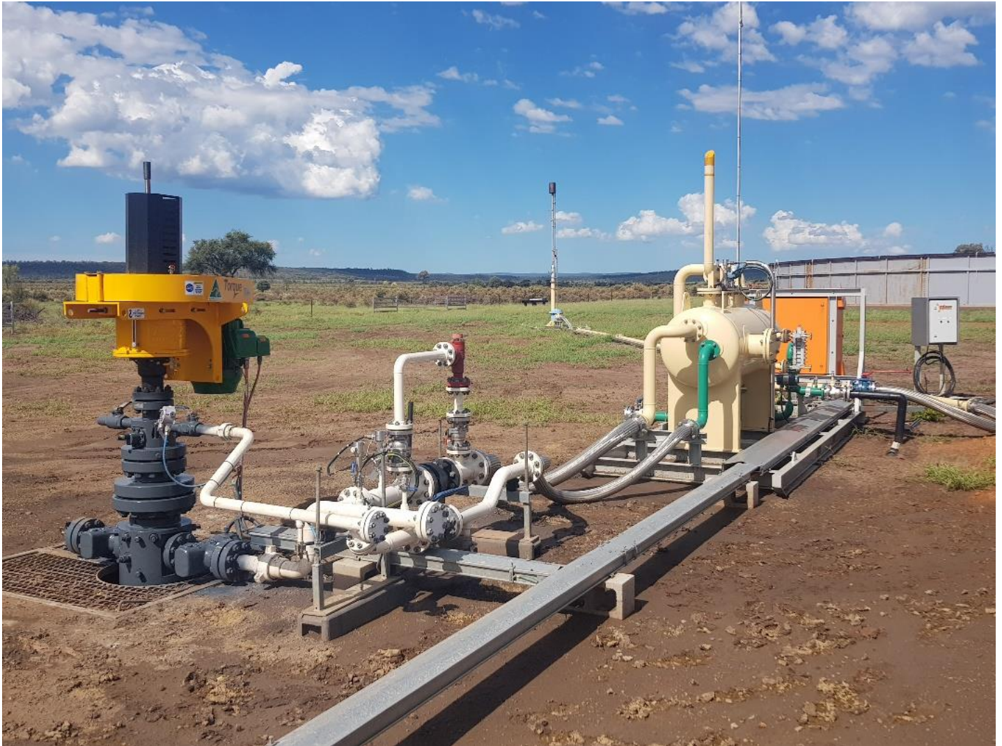
Figure 2: Mahalo East pilot flow package in place with wellhead and pump drive equipment on left, gas-water separator centre right and water storage tank and flare stack in the background.
