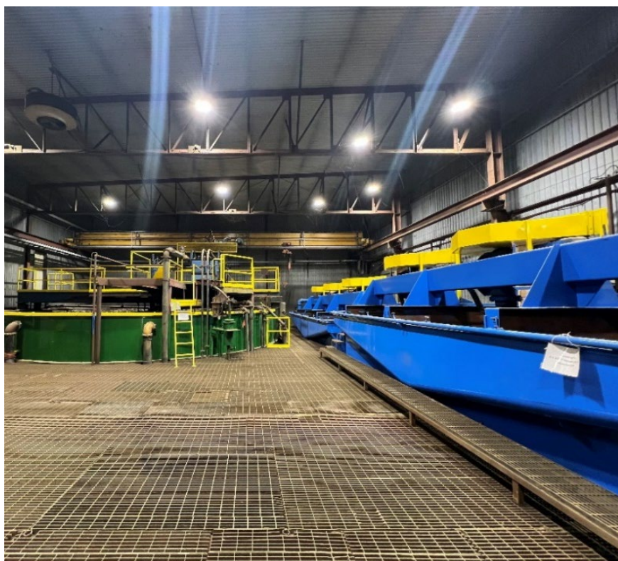
Figure 3: Processing plant infrastructure
