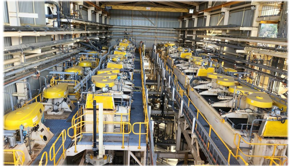
Outotec Flotation cells within plant building
