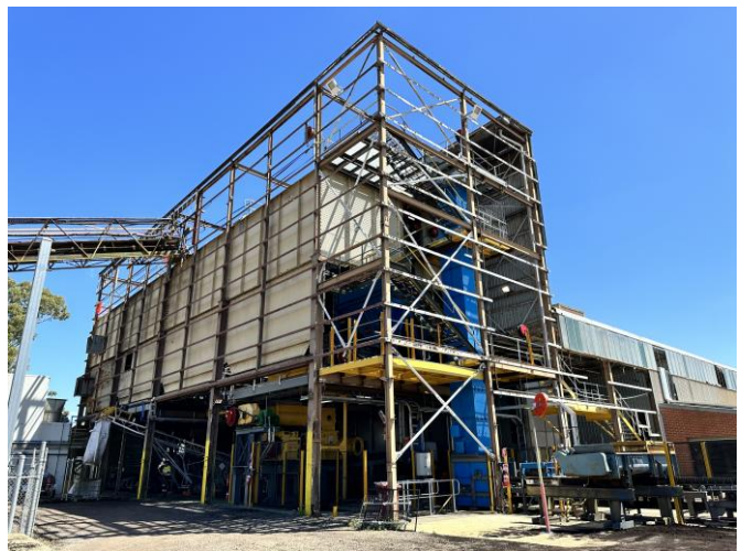
Photo: COLDry Demonstration Plant Bacchus Marsh, Victoria, Australia
