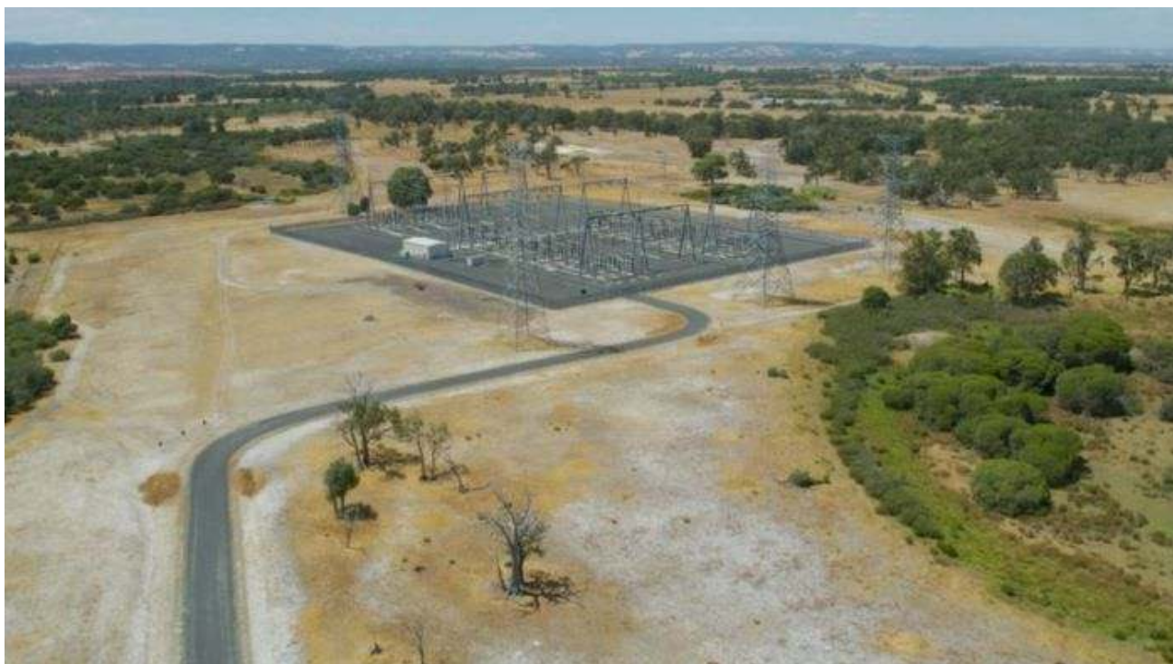
Image 4: Landwehr Terminal – 33/330kV
