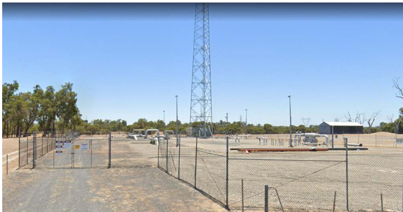
Image 7: DBNGP connection point
