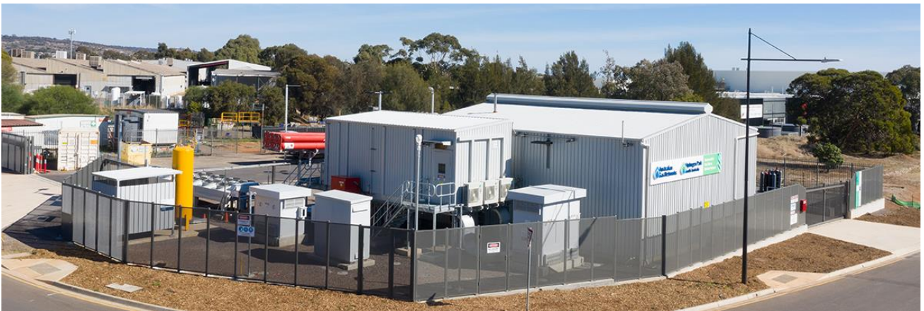
Figure 3: Hydrogen Park South Australia (source: AGIG)
