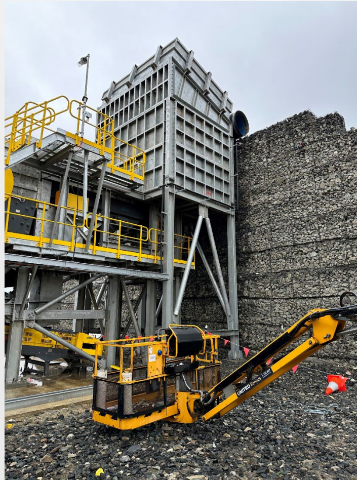
ROM Ore Bin and Primary Crusher
