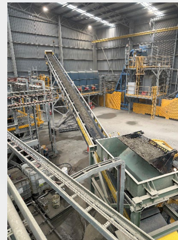
Concentrate Dryer and Magnetic Separator
