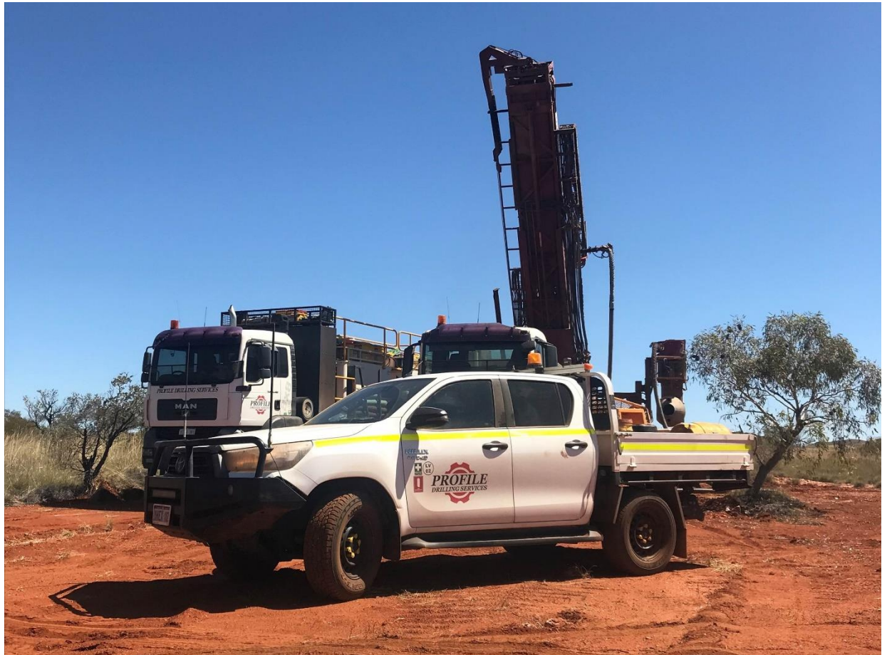
Figure 1. Profile Drilling Services mobilising to the Manna Lithium Project east of Kalgoorlie.
