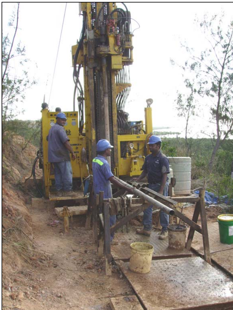
Figure 4. Drill rig (Exploration Drilling Services Pty Ltd) at FAD017A, Faddy's Gold Deposit, view towards the south west.
