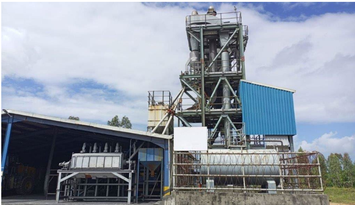
Figure 4 – Operational Flash Dryer and Screening Plant
