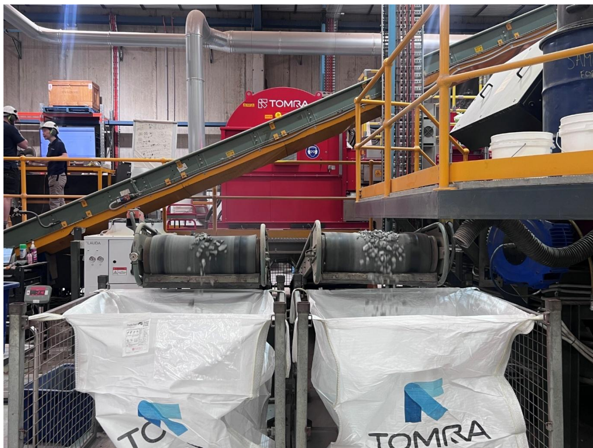
Figure 1 Orient material post ore sorting (LHS conveyor is product, RHS conveyor is waste)
