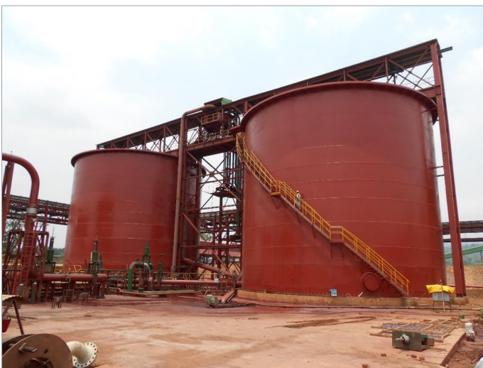
Typical tailings storage tanks with slurry intake box. (Image: WSP Australia)
