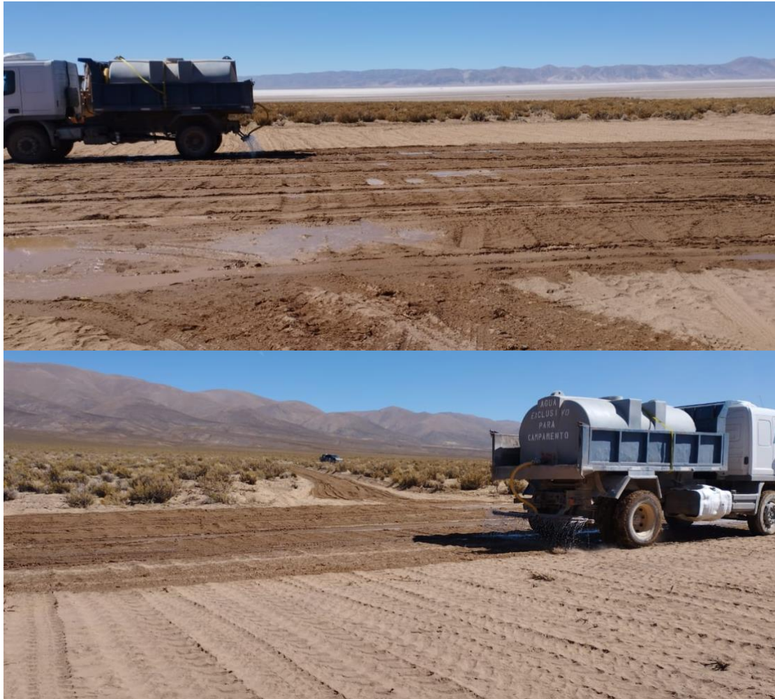
Figures 1 and 2: Site preparations for drilling first hole at Solaroz (Mario Angel Concession)
