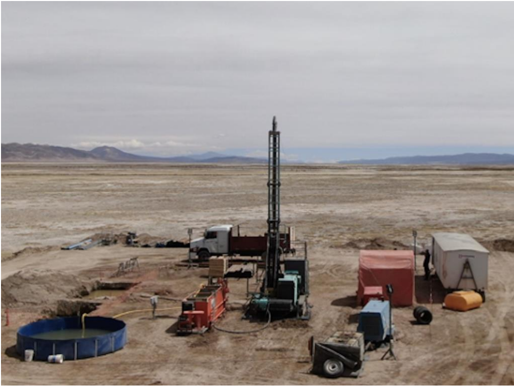
Figure 6: Second Diamond Drill Rig at SOZDD003, Chico I Concession on Olaroz Salar
