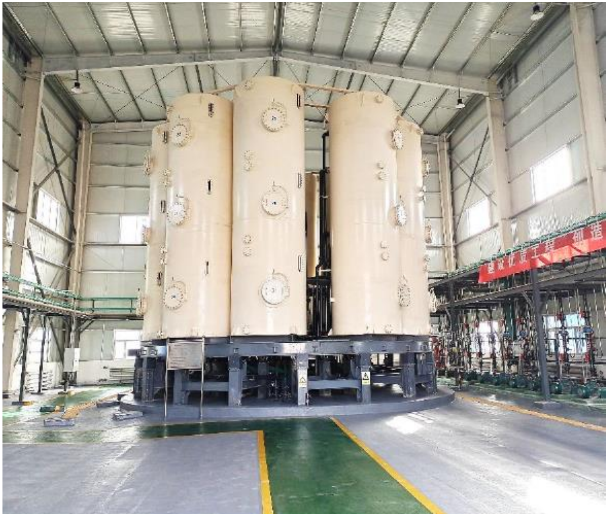
Figure 2: Lithium Adsorption Module of Lanshen Demonstration Plant, China
