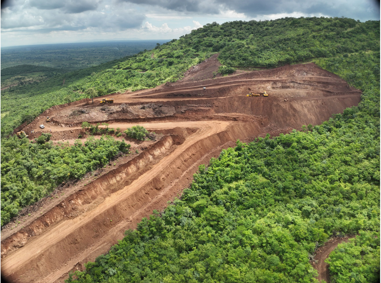
Picture 1. Earth works well underway preparing haul roads ahead of first blast.
