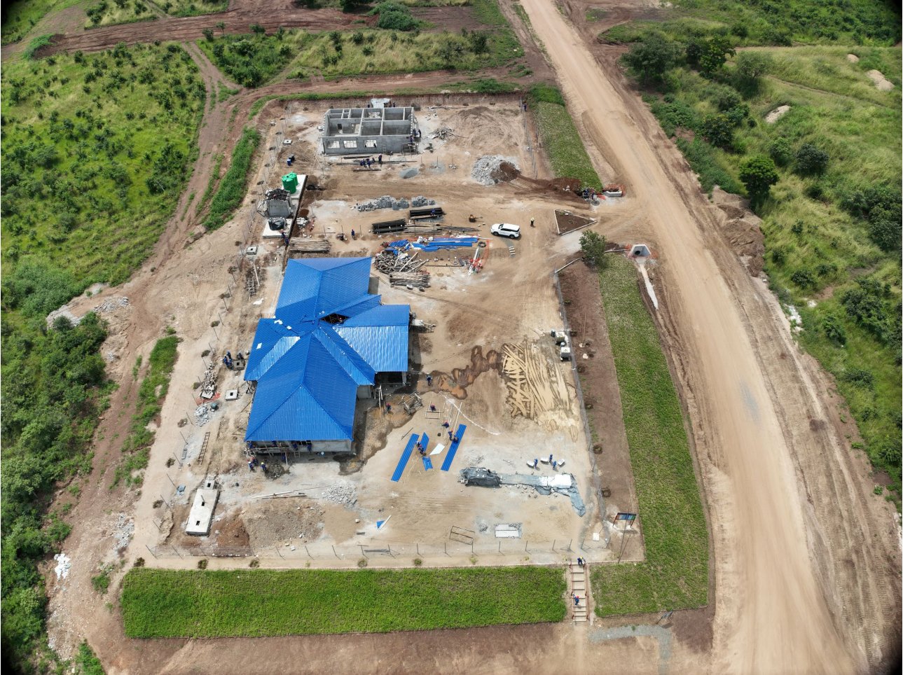
Picture 4. Aerial view of the site administration precinct under construction including the admin building and site medical clinic
