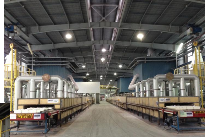
8 tunnel furnaces (88m long)
