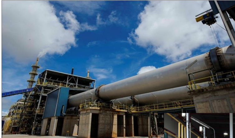
4 rotary kilns (60m long)
