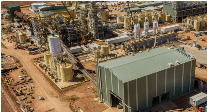
Concentrate Building and conveyor to the kiln; ready for kiln heating and production
