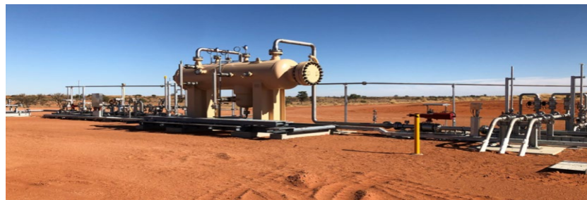
Vali -1 production separator/infrastructure
