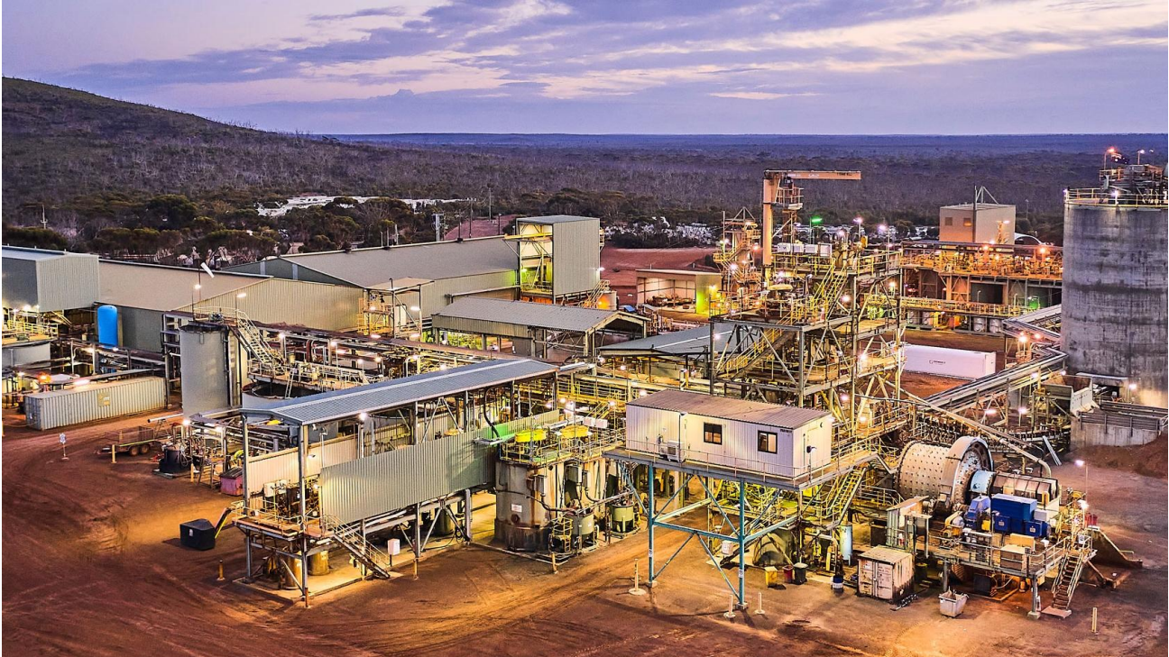
Figure 1: Existing CBC infrastructure with MREP plant and primary ball mill annotated
