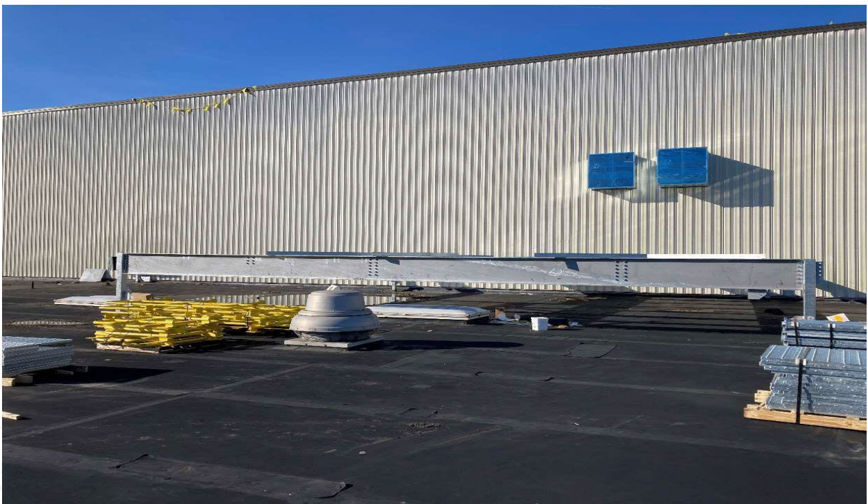
Figure 3: Roof AHU Platform
