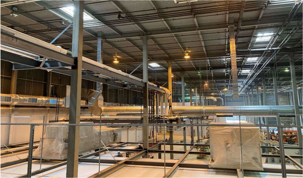
Figure 2: High Bay Ductwork and Insulation
