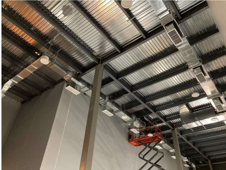
Figure 3: Anode Mixing room HVAC
