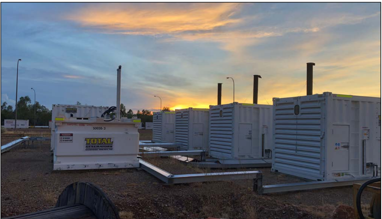
Figure 2: 4MW in diesel power generators delivered to site & installed for commissioning activities. Post commissioning, the diesel generator power forms the backup power system for ongoing operations (re-establishment of grid power connection underway).
