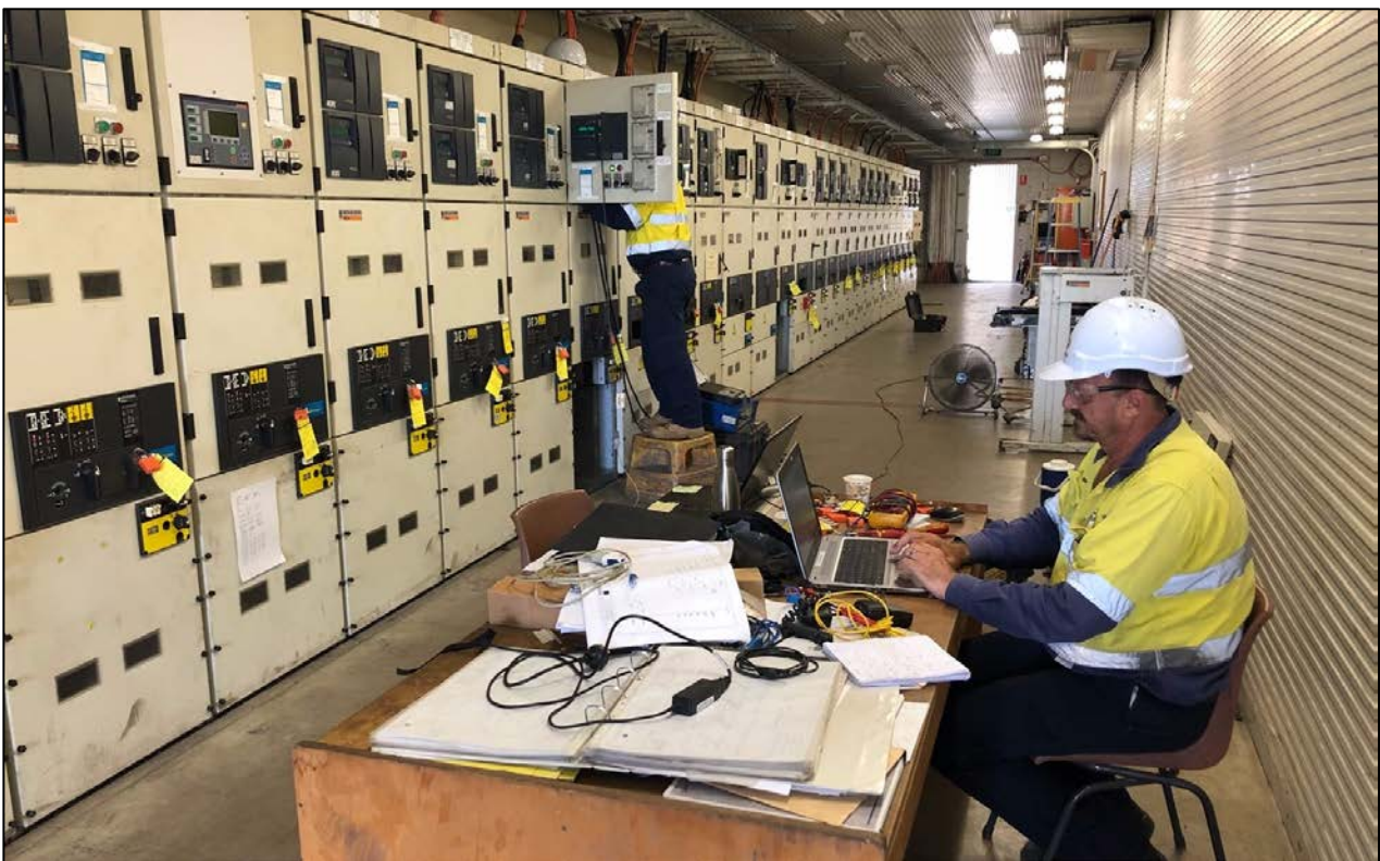
Figure 1: Sedgman and New Century employees undertaking re-energisation works of the Century mine electrical substation in preparation for commissioning activities
