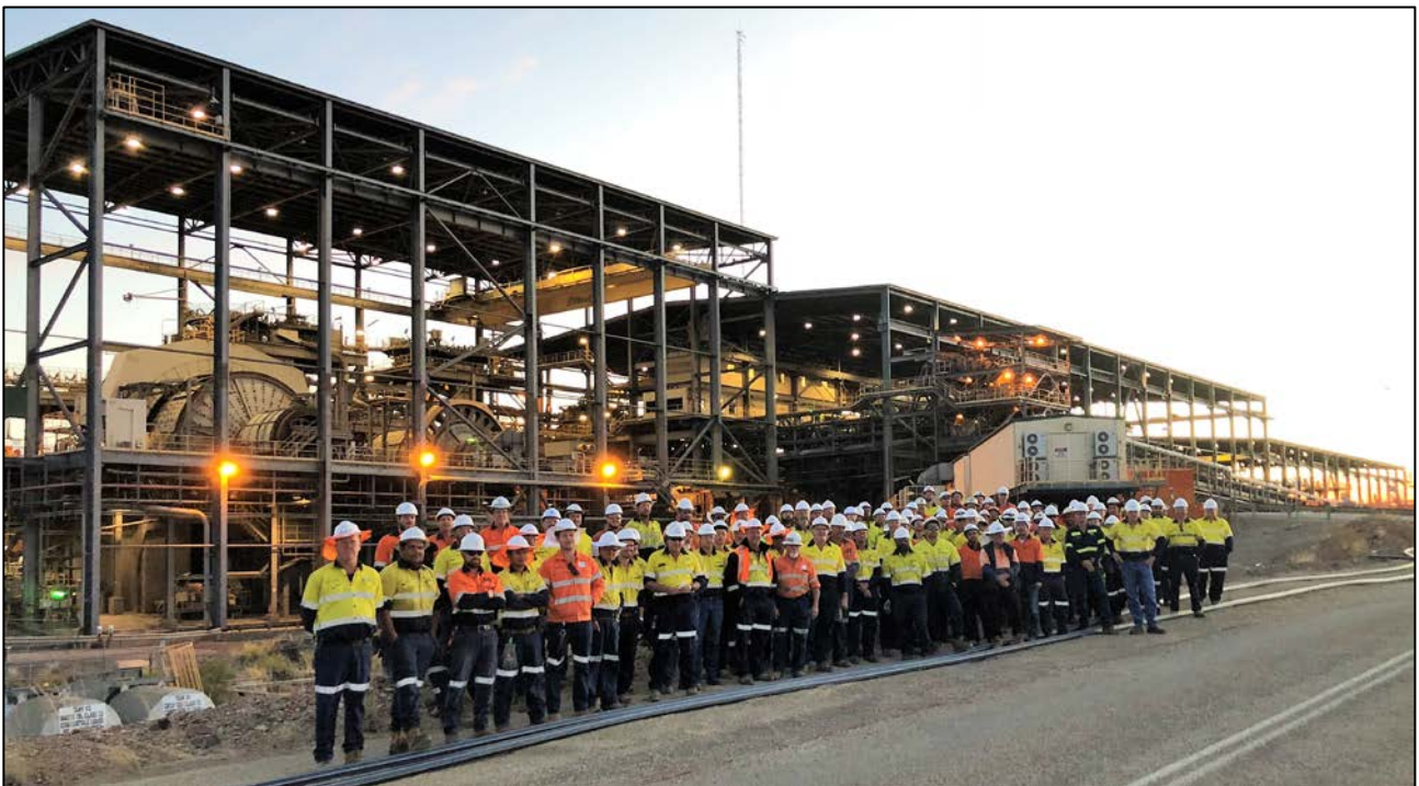
Figure 1: New Century and Sedgman site teams currently undertaking refurbishment and commissioning works
