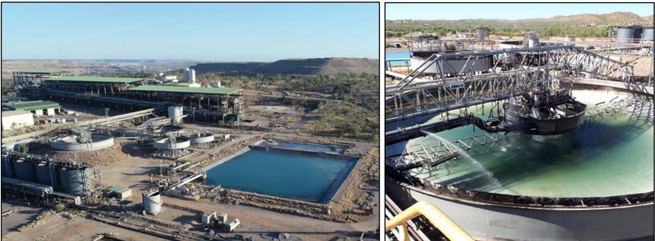
Figures 5 & 6: Process Water Dam re-established in preparation for water commissioning (left) and hydrostatic testing of the Tailings Thickener as part of initial commissioning activities (right)
