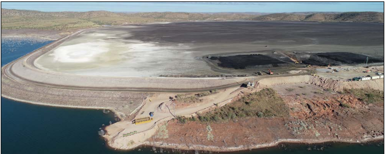
Figure 2: Overview of the hydraulic mining operations area in the SE corner of the Century Tailings Deposit
