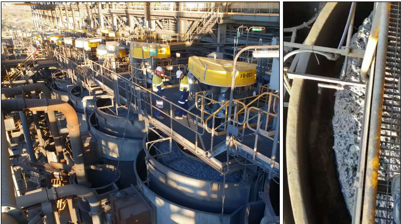
Figure 1: Zinc rougher concentrate production at the Century Processing Plant
