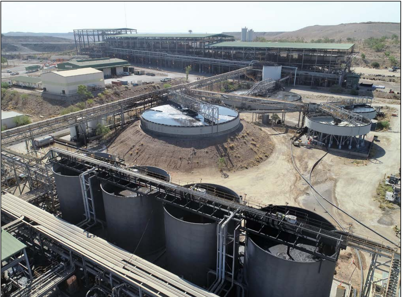
Figure 7: Zinc concentrate product in storage tanks and the zinc thickener at the Lawn Hill mine site, ready for pumping to Karumba
