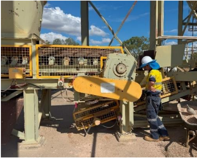
01-FE-02 Feeder Testing
