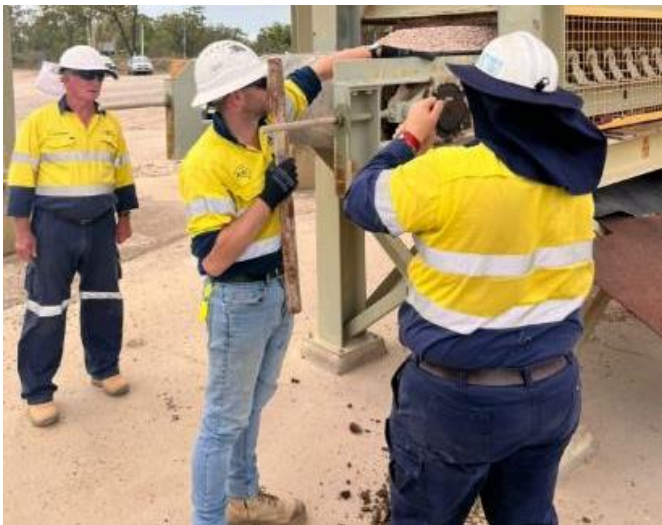
Tightening 01-FE-02 in preparation for emptying Fine Ore Bin
