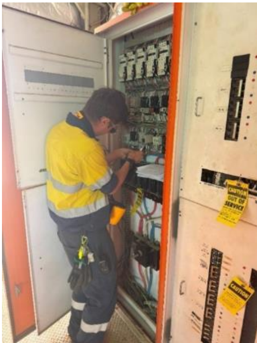
Distribution Board Testing
