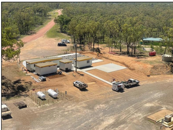
Overview of Administrative Area 13 th Jan 2025 with Main Office Block ETA 20 th Jan 2025
