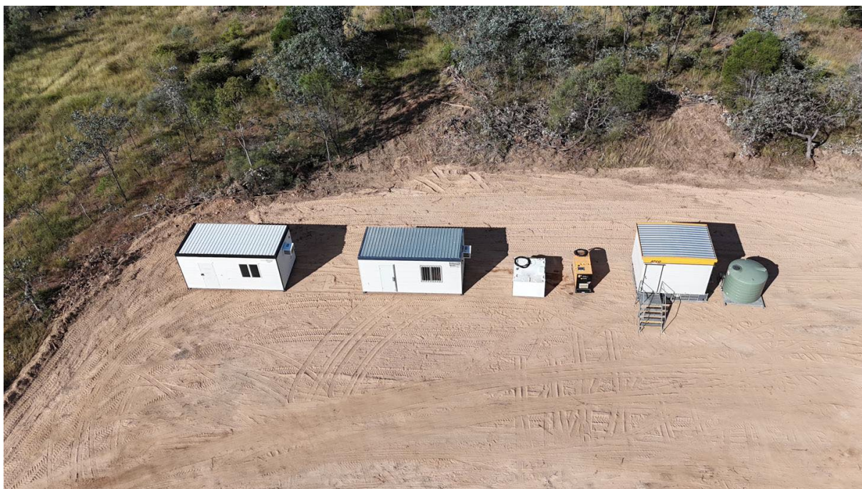
Figure 3: Podosky site establishment – site offices, generator and water infrastructure in place (22 April 2026)
