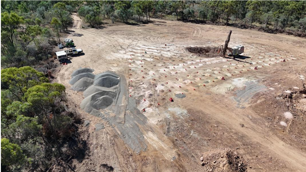
Figure 8: 277.5-004 Drill & Blast activities ongoing as part of second blast scheduled later in the month.
