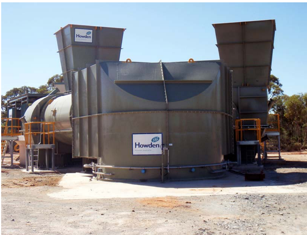
Figure 3: Deacon Ventilation Fan
