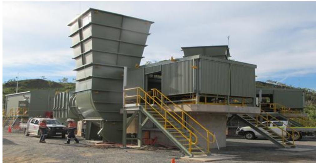
New ventilation fans at Savannah
