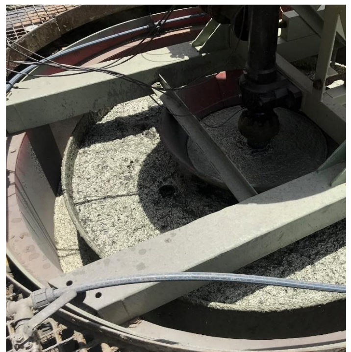
Photo 4: Flash Cell being recommissioned
