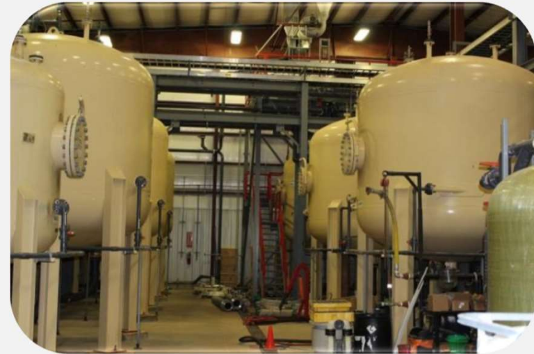
Lance Satellite Plant Ion Exchange System
