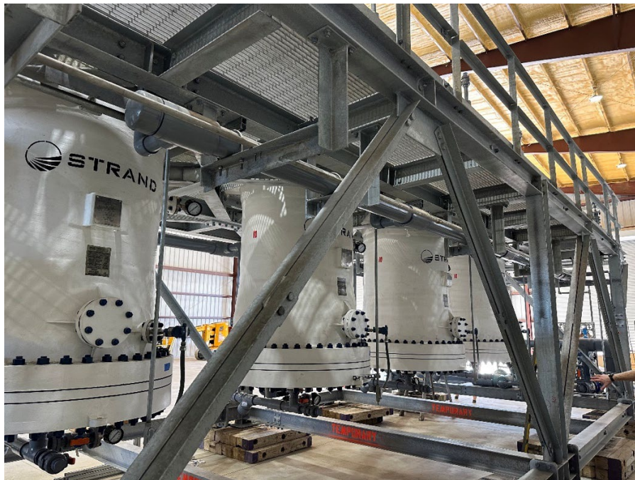
Figure 3: Close Up View of Prairie Lithium's four column Commercial Scale DLE Unit undergoing FAT
